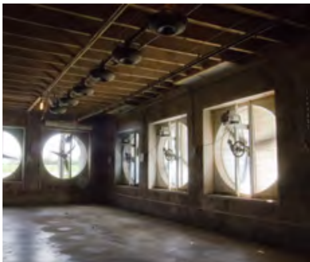
Mechanical ventilation uses fans, like those pictured above, to ensure that the house does not overheat.
